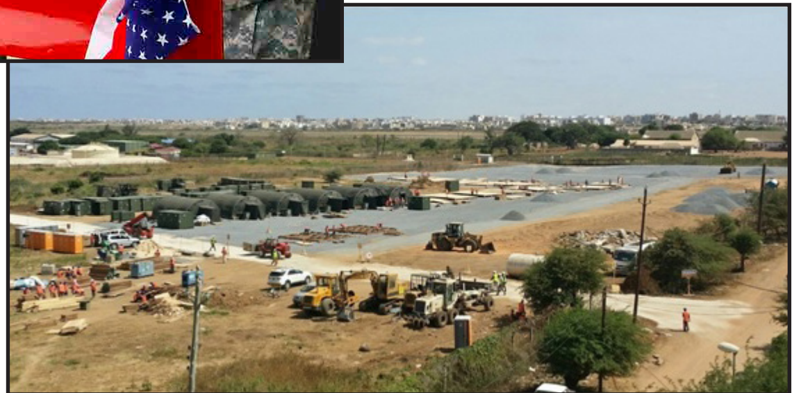
Construction of an Intermediate Staging Base in Dakar, Senegal, to support the Ebola response in 2014 (above)
